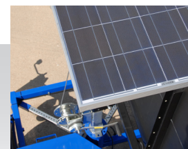
Solar panel system
