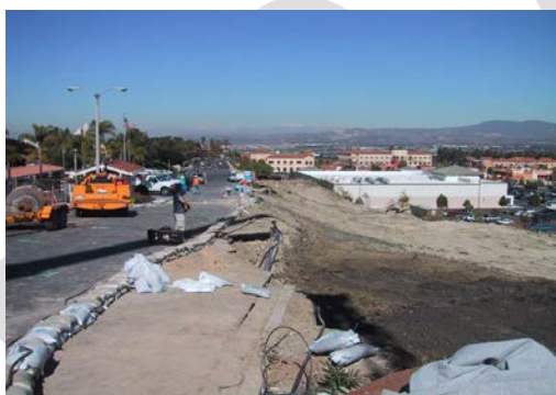
Looking north along Calle Sonora toward El Toro Road with the roadway damage visible at center-left (2004)
