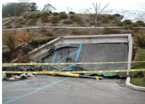
Looking southeast from the Home Depot Shopping Center with parking lot and slope damage visible (2004)
