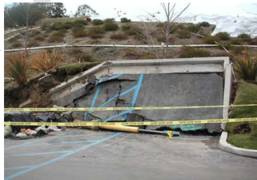
Looking southwest from the Home Depot Shopping Center with parking lot and slope damage visible (2004)
