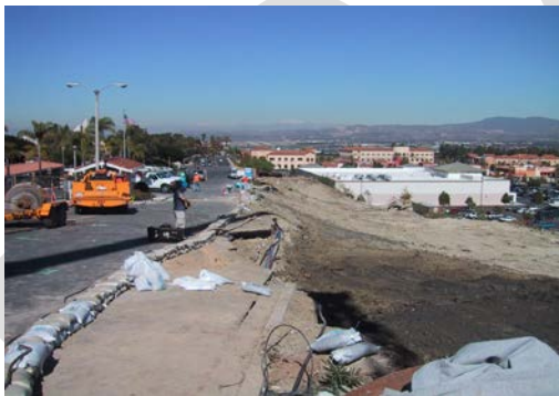
Looking north along Calle Sonora toward El Toro Road with the roadway damage visible at center-left (2004)
