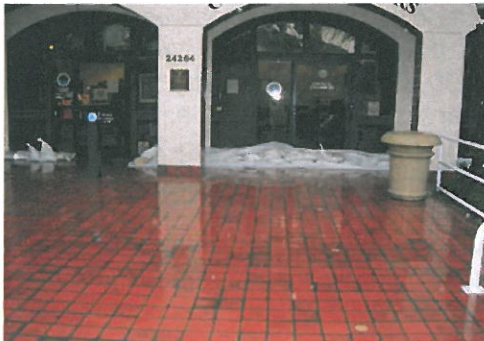
Sandbags were used to hold back rising water in front of the entrances to City Hall and the City Council Chambers
