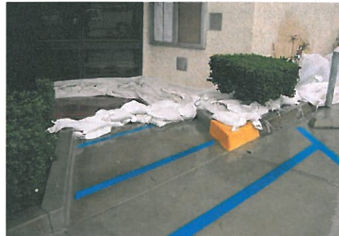
Water intrusion affected the emergency communications room at City Hall (located on the other side of this wall)
